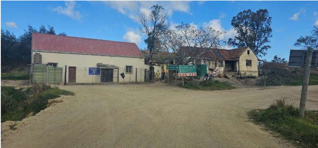
Photo 2 A building used for occasional religious purposes (left side) and a dilapidated dwelling that is illegally occupied. The photo was taken from the DR 1599 in a westerly direction.
