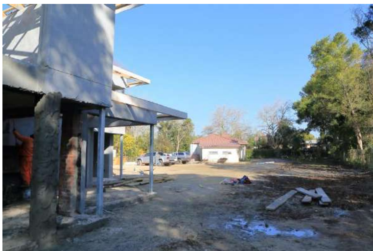
Photo W – Looking West from the 2 nd dwelling towards the house to be demolished.
