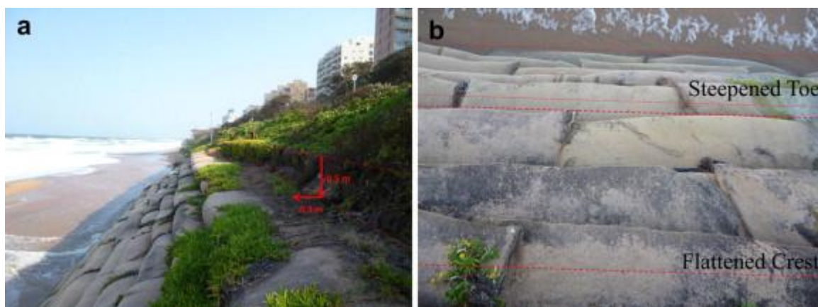
Figure 8. A bag seawall in Umhlanga Rocks (29/08/2011) showing (a) the movement of the seawall relative to its original position and (b) the steepening of the seawall toe and the flattening of the seawall crest 21 .
