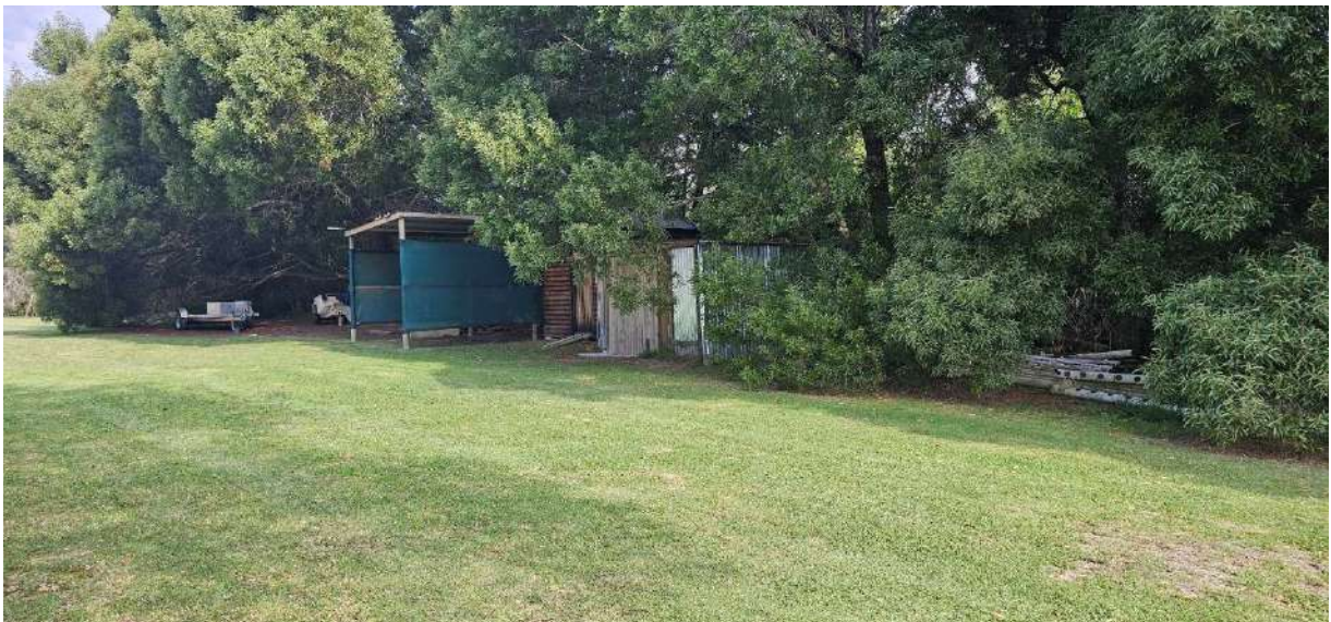
Photo 7 Structure used as carport and shed on the western side of the erf. These structures were erected over the building line by previous owners with slight modifications/addition by current owner and a relaxation is therefore required. The photo was taken in a south-westerly direction. Also note the dense vegetation behind the structure on the erf boundary.
