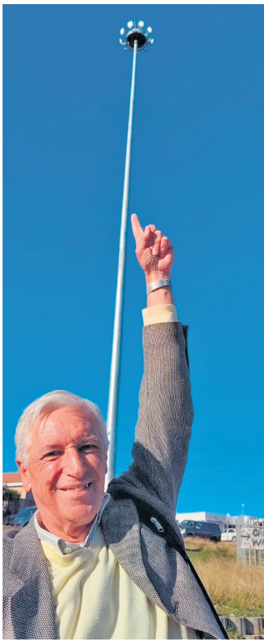
Mayor Leon van Wyk says the installation of these high mast lights is expected to yield safety.
