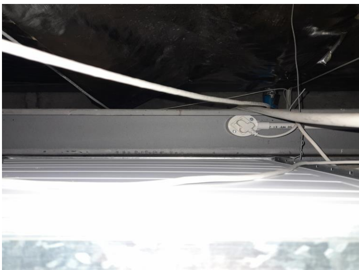
Image C: Ceiling view image of the office light.
